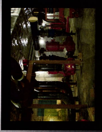
CHILLED WATER PUMPS AND PIPING
